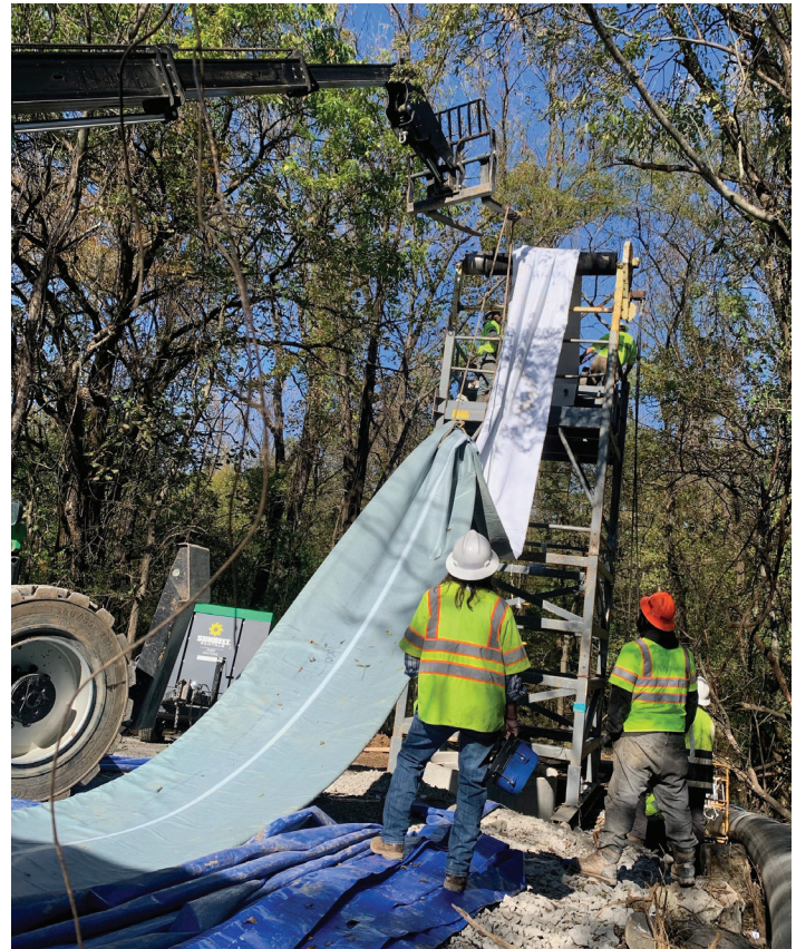
Crews insert a liner that will make a defective underground pipe new again. This method minimizes digging and pipe replacement and extends the life of existing infrastructure.
