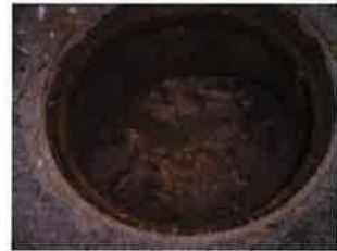
Sewer line blockage from grease.
