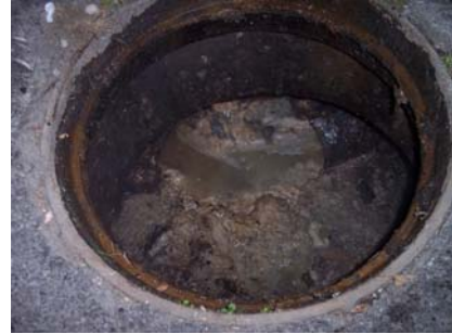
Sewer line blockage from grease.
